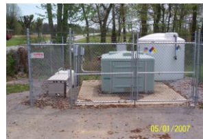
COMMERCIAL LIFT STATION
