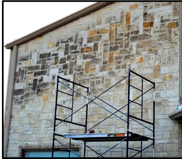
Figure 2: Left (N.W.) side of Texas limestone church stained by mold and pollutants prepared for deep cleaning.
