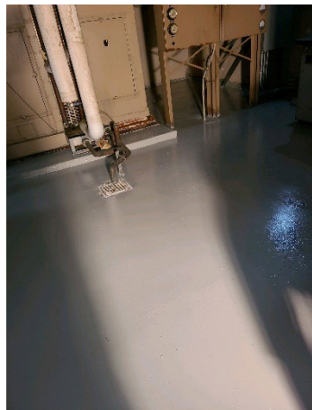
Figure 1: NewEraStrip™ Extreme Strip™ used to strip then glazed with NewEraSeal Wonder Walk.
